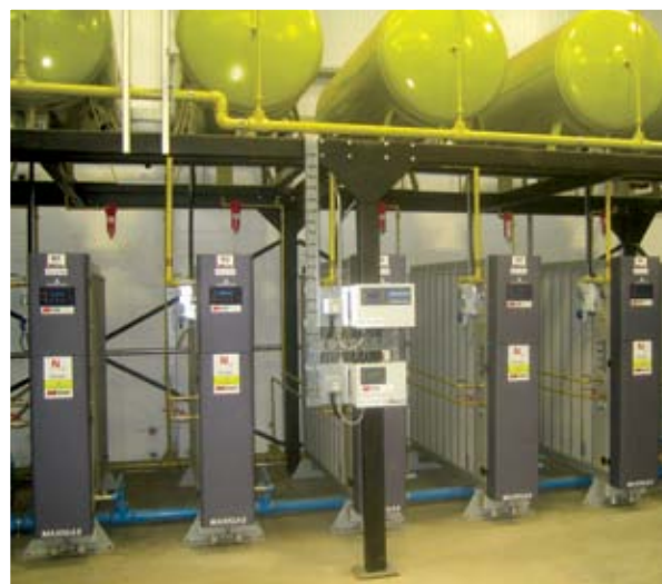
A six bank MAXIGAS installation. (Five generators in view) satisfy the peak demand, each capable of supplying 20% of the output. The banks cascade on and off load as the flow varies with factory production requirements. This saves significant energy costs during low flow periods, in the form of lower compressed air demand. The sixth bank provides 100% back-up and allows for 100% up-time during maintenance.
